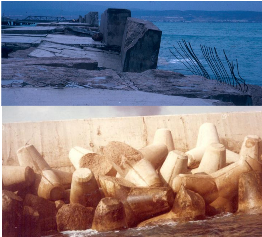
Figure 6 Photos of Arzew el Djedid breakwater damage. Above, most damaged sections and below, section with settlement of entire armour layer and broken units.
