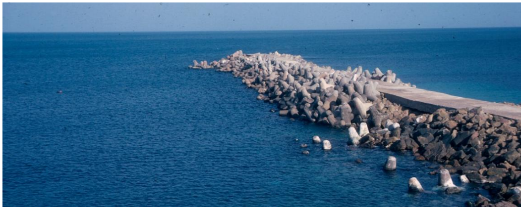
Figure 2 Damaged tetrapod breakwater in El Kala, Algeria.
