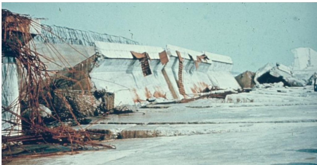
Figure 4 Sines breakwater failure seen from behind the superstructure.
