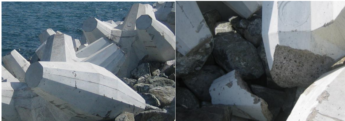
Figure 14 Example 2: Core-Loc breakwater with approx. K_D=16 . Note settlement of entire armour layer creating gap at wave wall and some breakage.
