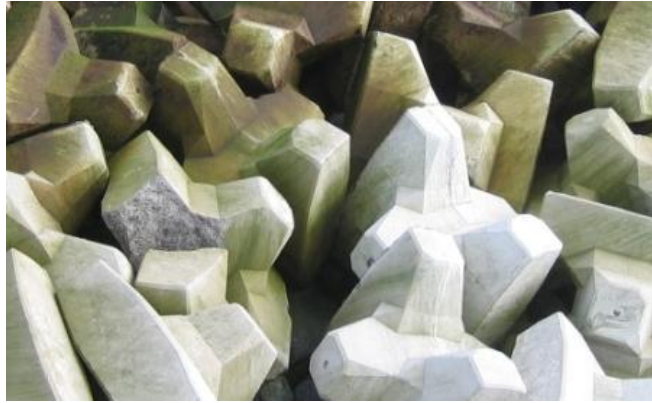
Figure 13 Example 1: Accropode breakwater with approx. K_D=15 after exposure to design event. Note broken units and openings, non-interlocking units.
