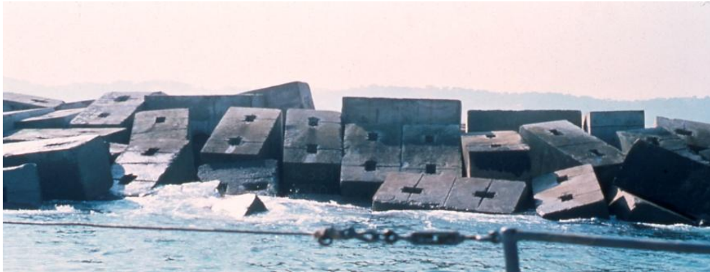
Figure 1 Example of breakwater built in the 1930'ies and armoured with large rectangular blocks.
