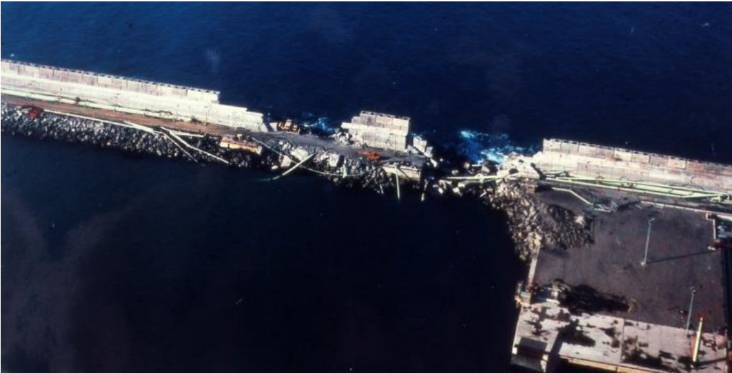
Figure 7 Bilbao breakwater cross section and photo of damage from the port side.
